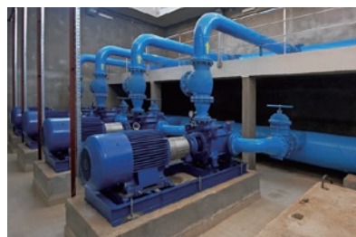
Building water pumps
